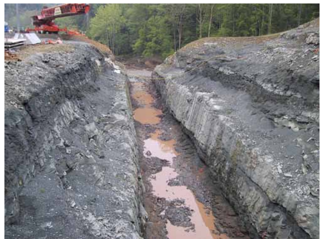
Figure 7–10 Presplitting in the bypass and auxiliary spillway at Hughes River Dam in West Virginia
