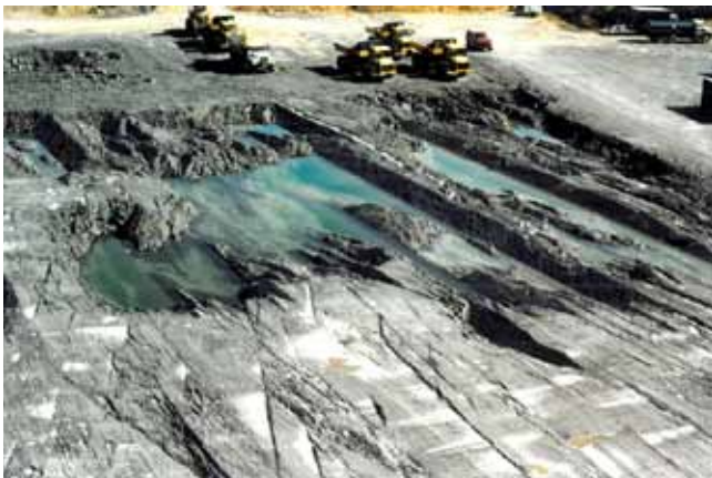
Figure 7–12 Results of overblasting in an auxiliary spillway
