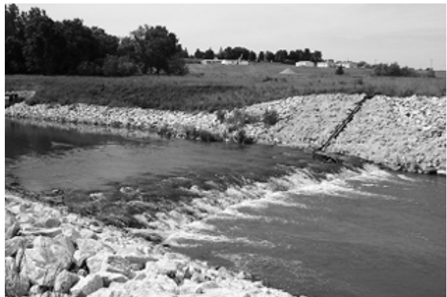
Figure TS3B-5 HCA steel sheet pile weir with riprap and cement grout that protects a large sewer main for the City of Denison, IA
