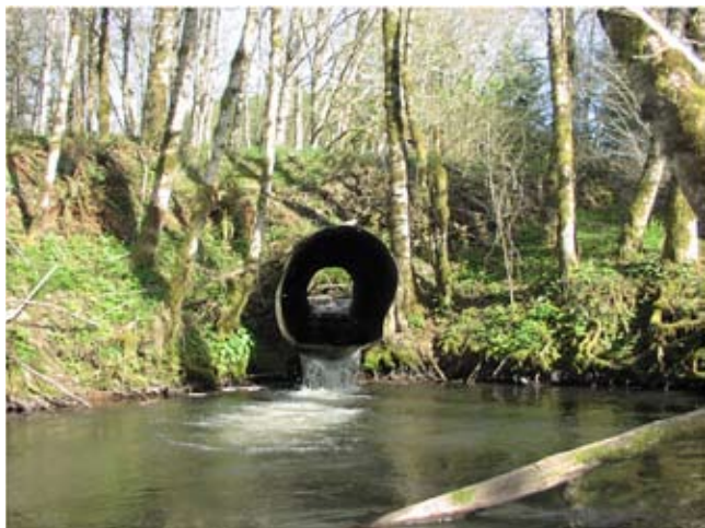
Figure TS14Q-3 Forest road culvert acting as fish passage barrier (Photo courtesy of Christi Fisher)
