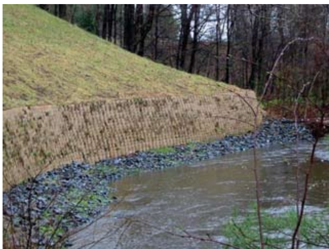
Figure TS14D-17 Geocell earth retaining structure (Photograph courtesy of Carl Gustafson, NRCS MA)
