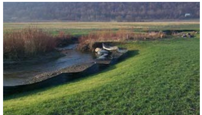
Figure CS7-7 Completed section of streambank stabilization to include J-hook vane and intentional point bar, Spafford Creek, NY
