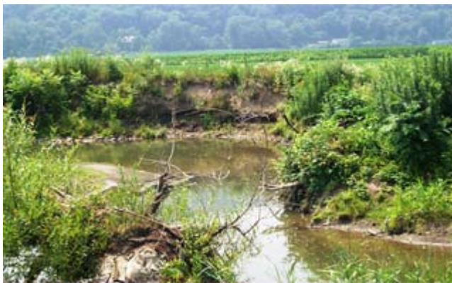
Figure CS7-1 Typical picture of streambank erosion along entire project reach south of Sawmill Road, Spafford Creek, NY
