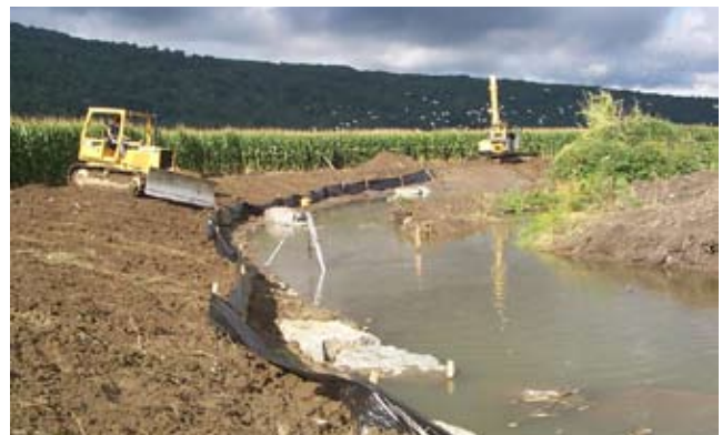
Figure CS7-5 J-hook vane installed and final grading of streambank followed by seeding and mulch, Spafford Creek, NY
