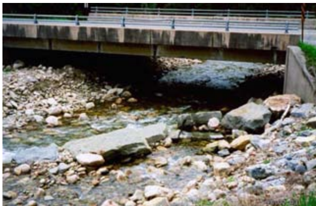
Figure CS6–15 Vane with a tip-out vane rock due to the scour from a gap hole
