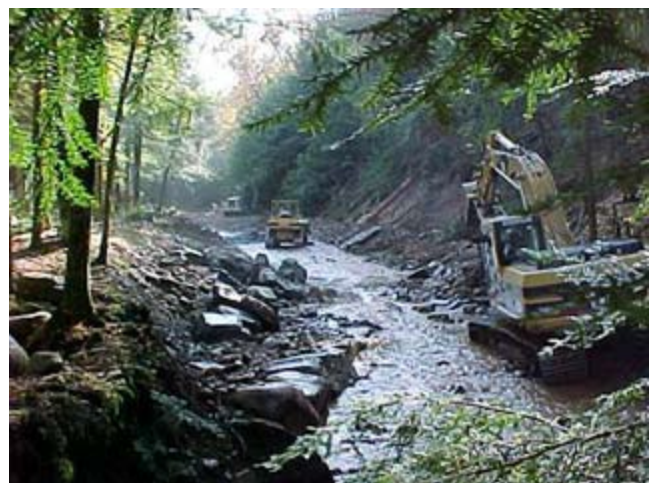
Figure CS6–19 The open heart surgery approach, working with heavy equipment in the channel of Big Bear Creek
