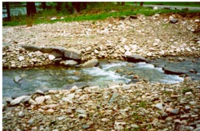
Figure CS6–16 Tip-out due to scour from a suck hole
