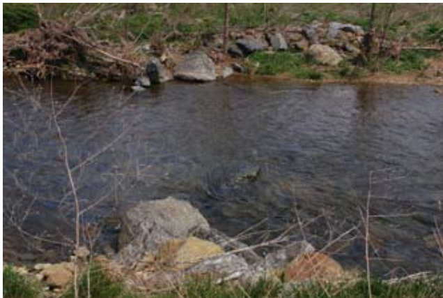
Figure CS5-12 Weir #7, April 2004, after Hurricane Isabel
