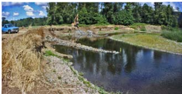
Figure CS17-7 Looking downstream at initial installation of two barbs before bank shaping, during low summer flows ( Photo courtesy of Scott Wright )
