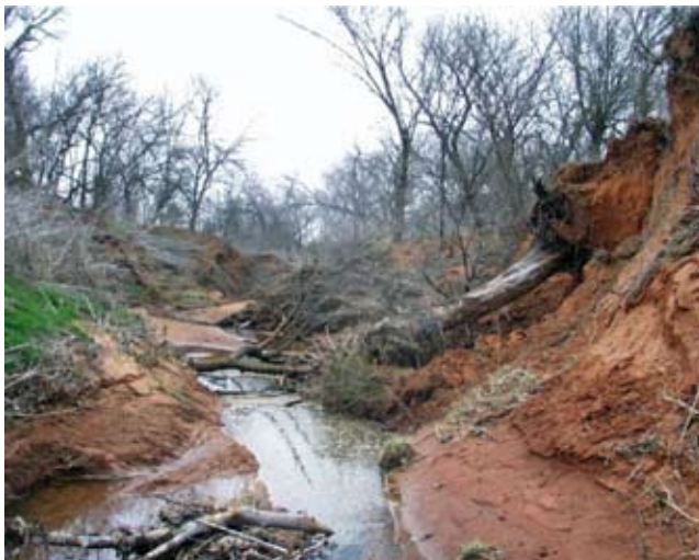
Figure CS16-3 Streambank erosion prior to the project
