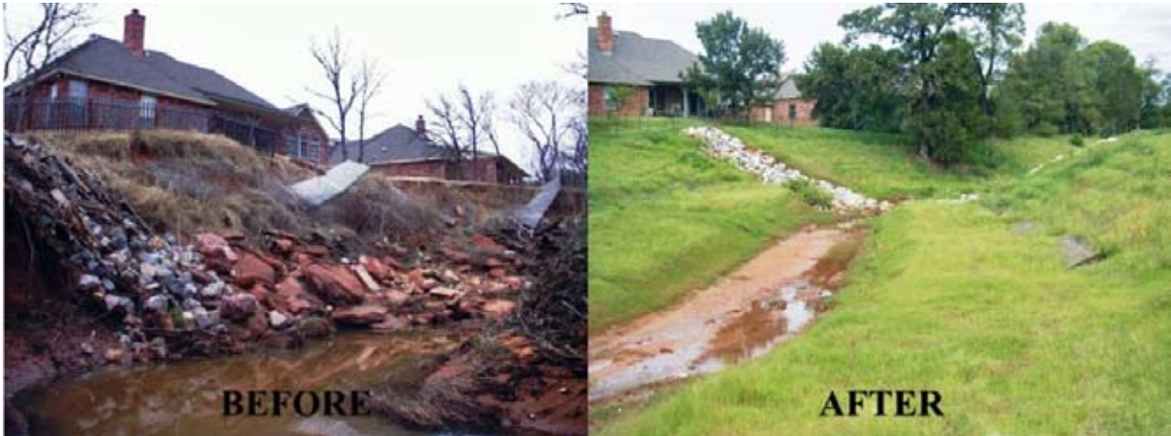
Figure CS16-9 Eroding channel prior to construction, and after project implementation; house and property lines imposed restrictions on the design
