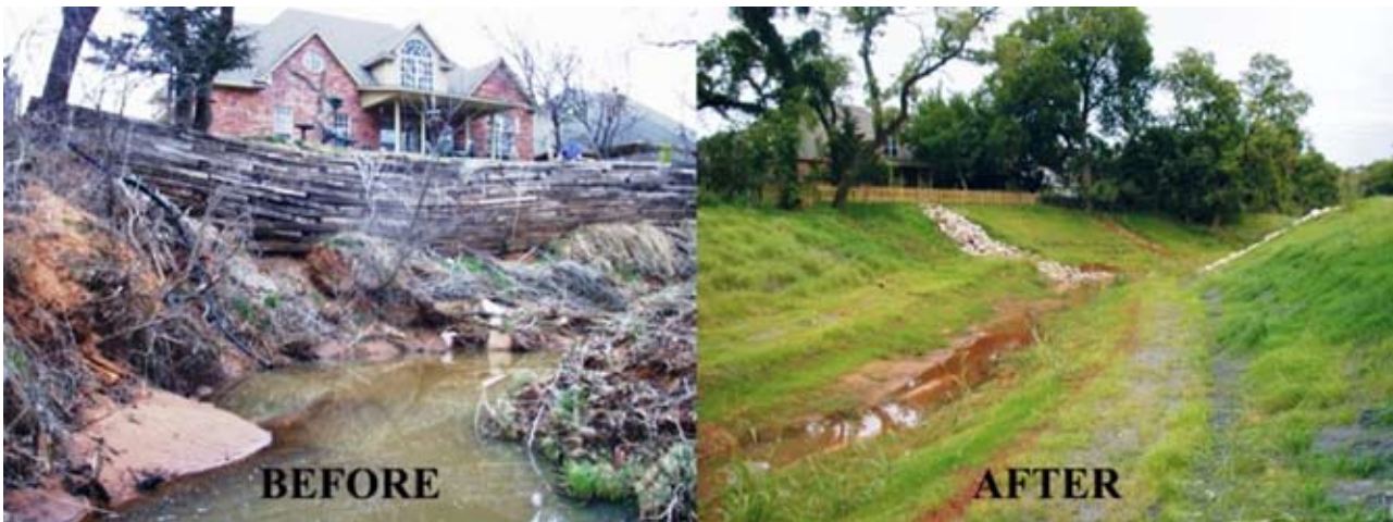
Figure CS16-10 Eroding channel prior to construction, and after project implementation; house and property lines imposed restrictions on the design
