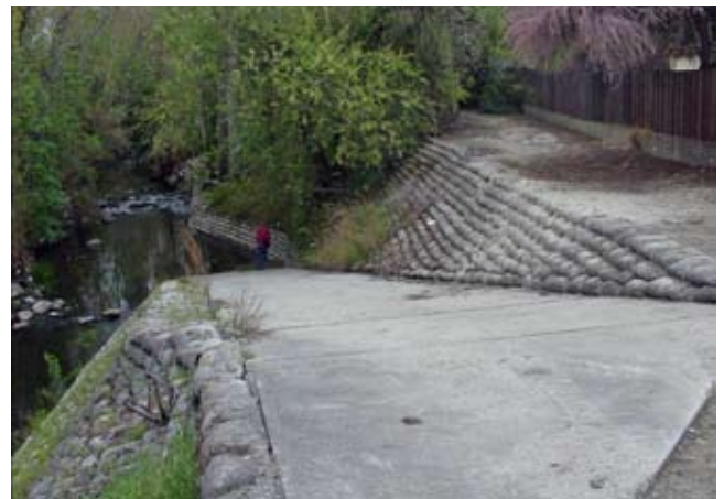
Figure CS15-1 Damaged access ramp and wall
