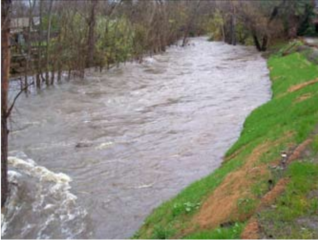
Figure CS15-10 Inundation of the restored slope
