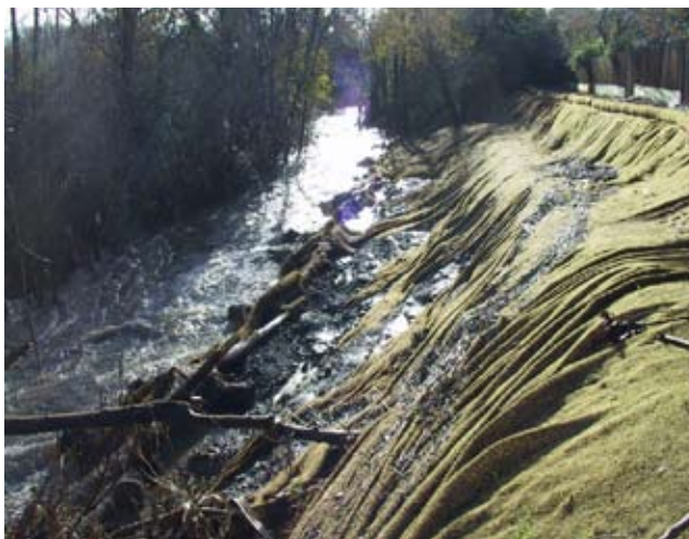
Figure CS15-3 Damaged streambank following a 5-year frequency event in December 2002
