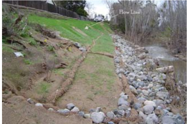
Figure CS15-11 Flow line after a storm in January 2004
