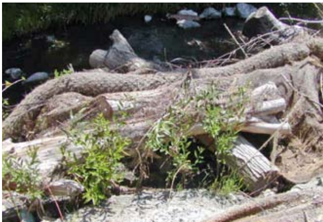
Figure CS15-4 Evidence of scour and exposure of the log structures
