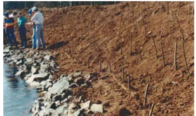
(b) 1992, after installation of live stakes. Note the fascine just above the toe rock.
