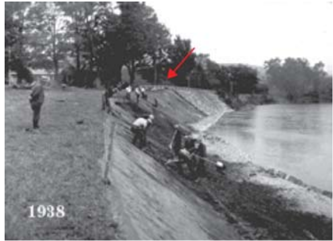
Figure E-5 Winooski River, VT, during construction in 1938. Note the work being done by hand.
