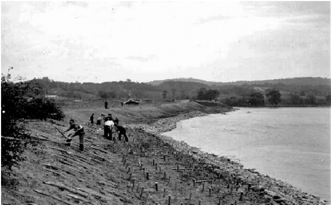
Figure E-1 Workers installing live willow stakes and brush matting on a terraced streambank, Winooski River, VT (September 1938)
