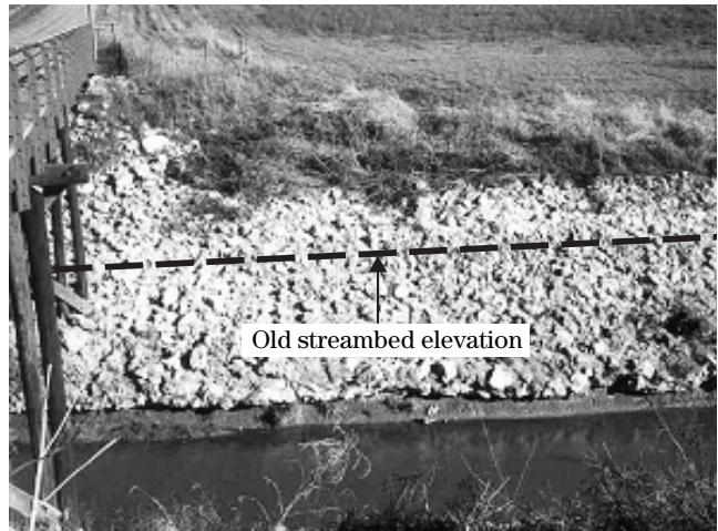
Figure TS3B-4 An NRCS bank stabilization site that did not include streambed stabilization, (Page County, IA)
