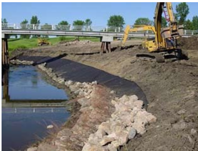
Figure CS11-17 Rock toe being placed over geotextile. A layer of live willow branches is visible within the rock toe.
